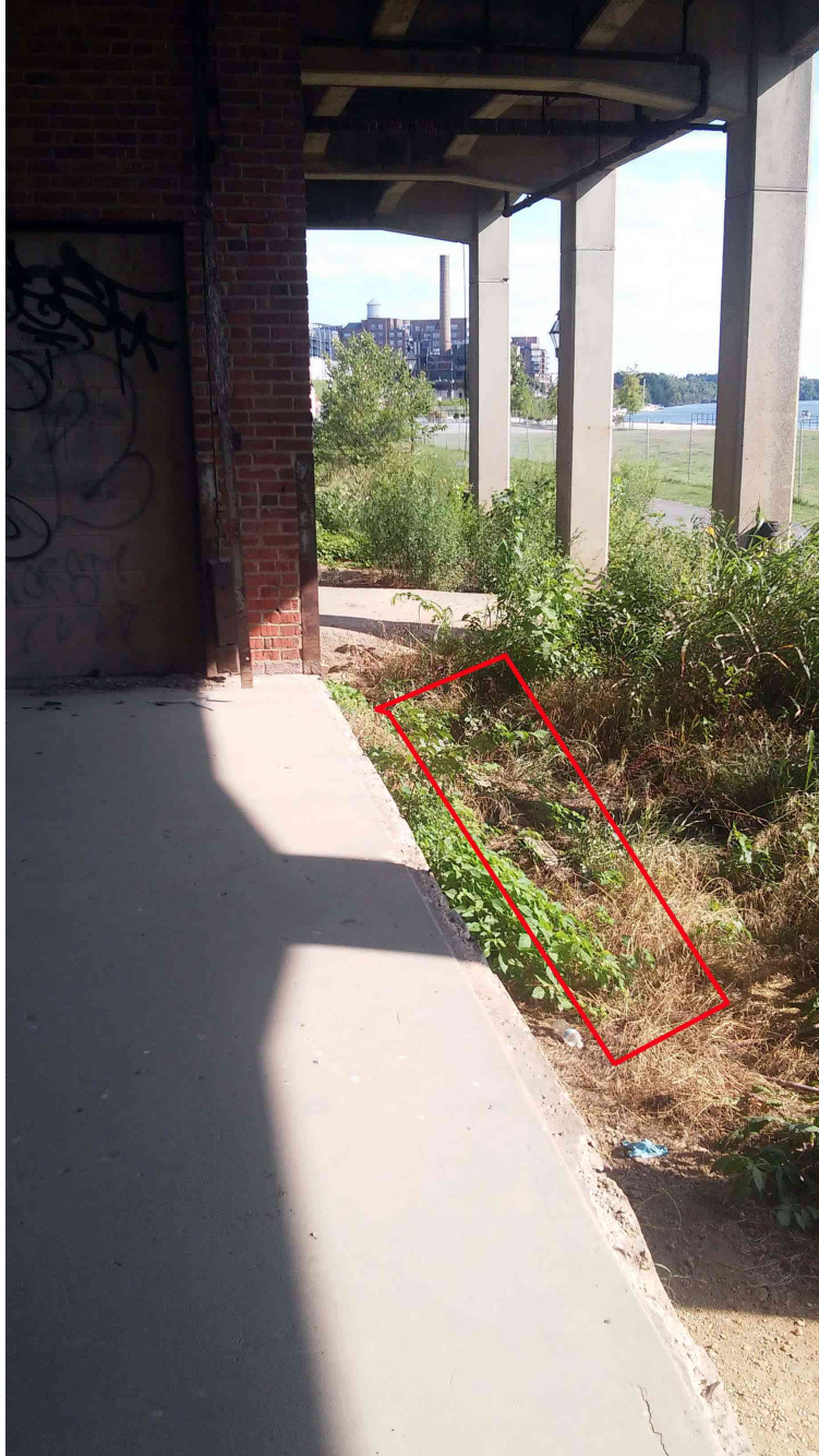
Railroad tracks still extant under the first bay of Terminal beside the loading dock and elevator.
