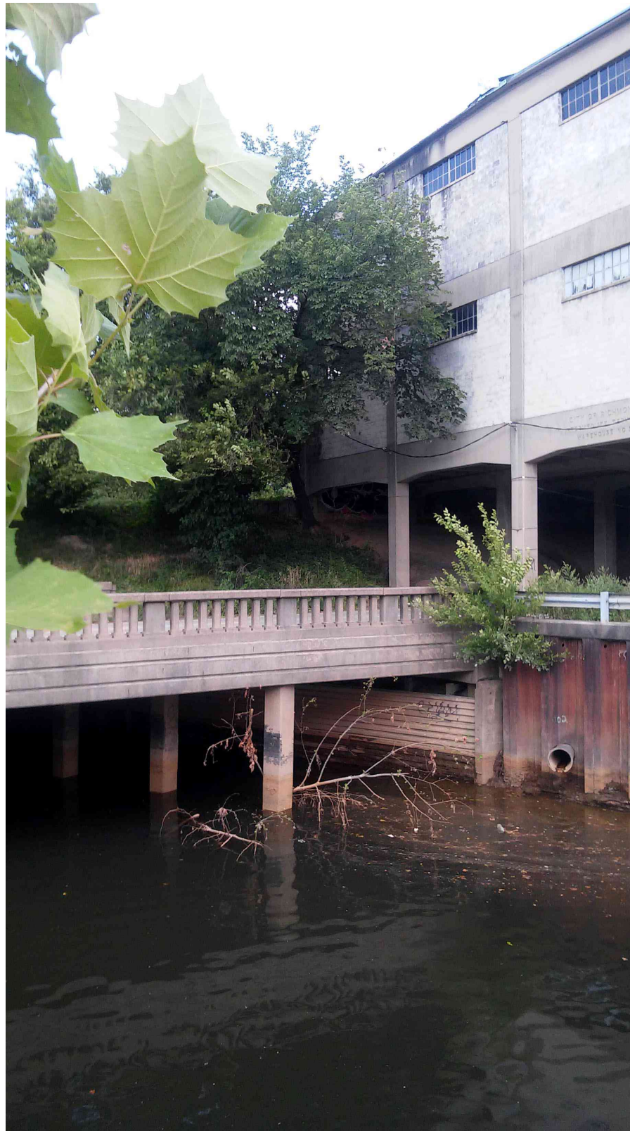
Water Street Bridge at Gillies Creek was built in 1938 as part of the same harbor improvements as the Terminal, probably with the same Public Works Administration funding. The bridge contributes greatly to the integrity of the setting of the Terminal.
